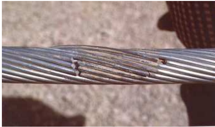
Fig 2.1 typical broken strand due to aeolian vibration after removal of suspension clamp.
